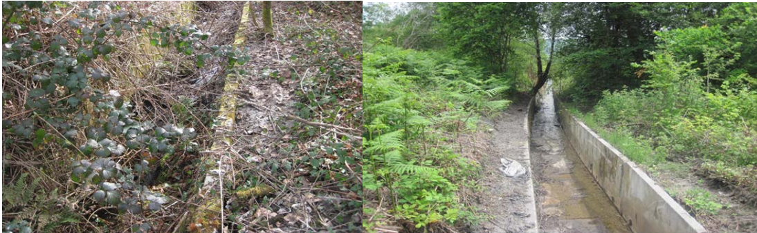
Site photographs taken on site to demonstrate the effective clearance of a tip concrete drainage channel
